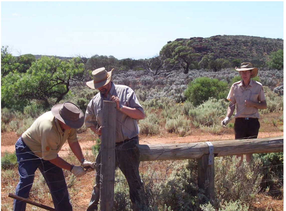
Lance Dean, John Carter and Clint Garrett working on repairing a section of fence in the north west corner of the Park during the December Working Bee.
