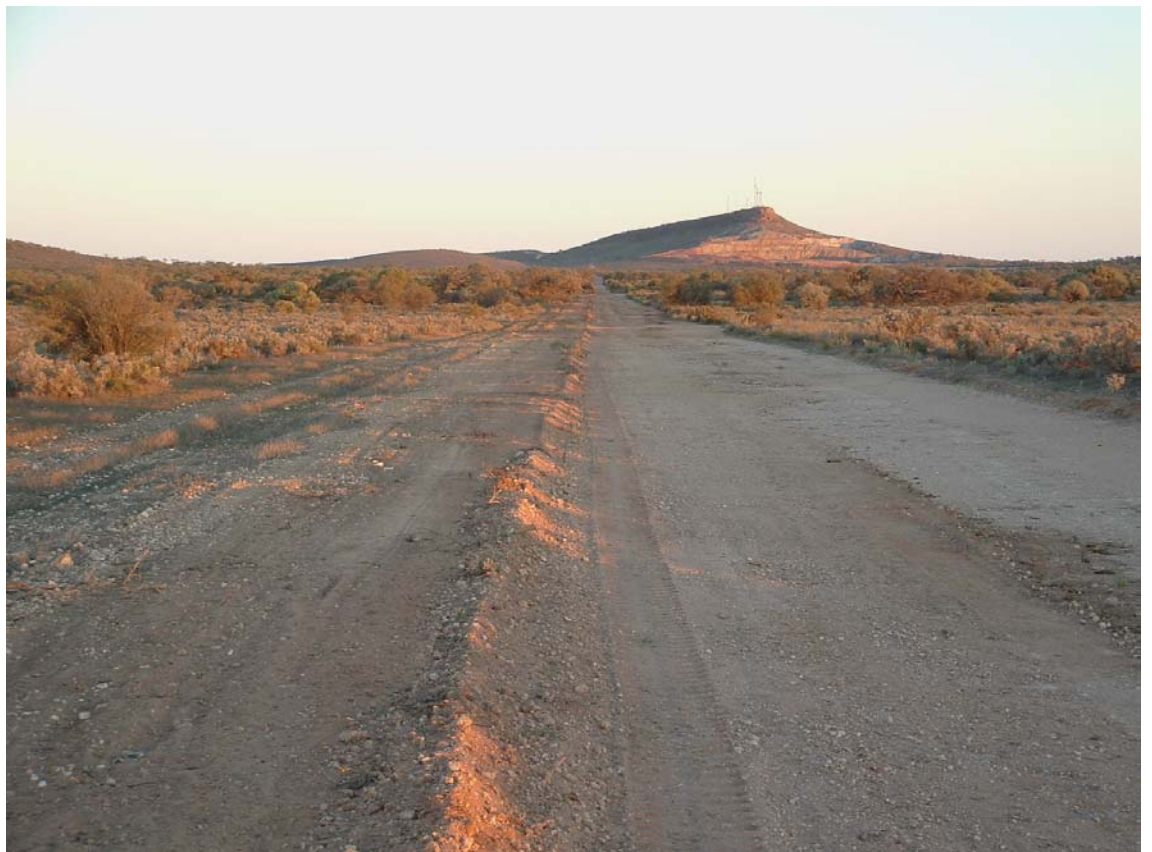
This photo shows the western boundary to the new section of the Park. It has been cleared by Brambles, paving the way for the installation of a new fence along the western boundary.
